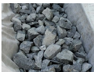
> Coarse untreated gravel, in chippings of size 60-100 mm, encased in a geotextile
